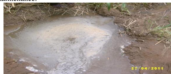
Plate 3. Leakage from the main line
