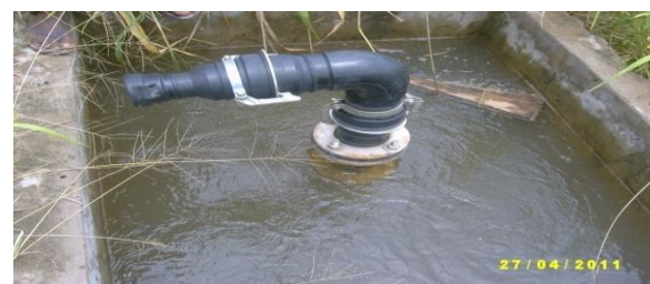
Plate 4. Leakage from hydrant joint
