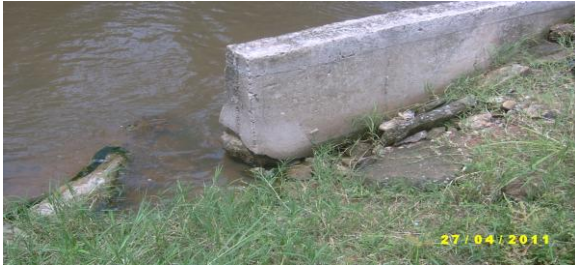
Plate 6. Leakage from the control
