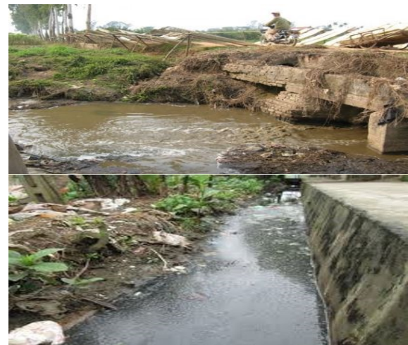
Fig. 3. The current state of the drainage channels in the commune
