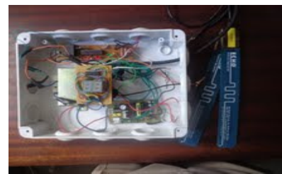
Fig.2. Soil moisture based irrigation controller circuit board and the sensors
